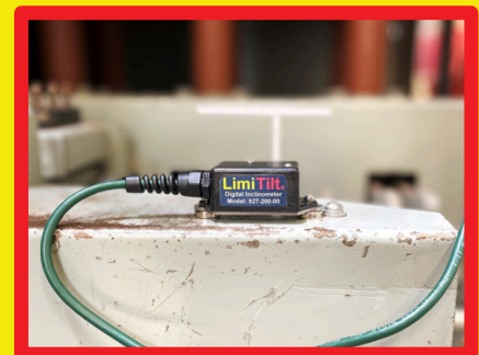
LIMITILT DEVICE SECURED TO BREAKER BY MAGNETS
