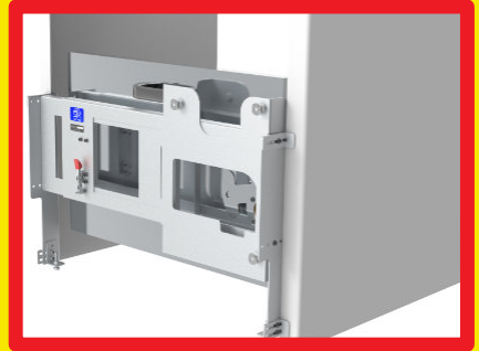
SPANNER BAR PLACED ACROSS BREAKER FACE
