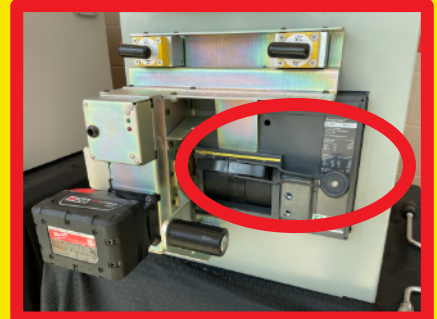
ROC WITH BATTERY ON BATTERY BLOCK AND BREAKER HANDLE MOVED OUT OF THE PATH OF MANIPULATING LEVER
