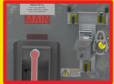
SDB SUSPENDED FROM CUBICLE USING SWITCHING MAGNETS
