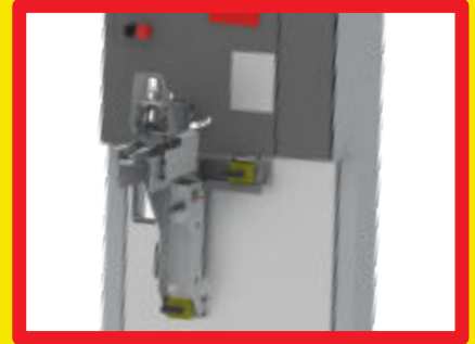
SDB ALIGNED WITH AND LOCKED IN PLACE ON CUBICLE USING SWITCHING MAGNETS
